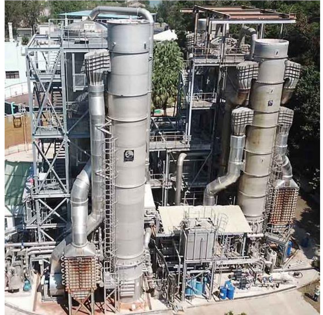
Organics Group: Thermal stripping ammonia recovery
