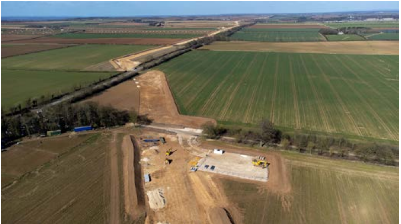
Part of the innovative Strategic Pipeline Alliance , the biggest drinking water grid program in the U.K. in a generation, we're supporting Anglian Water's key strategic aims to make the East of England resilient to the risks of drought and flooding and to be a net-zero carbon business by 2030.
