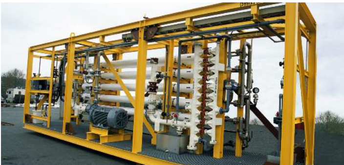
A larger unit with automatic control.
