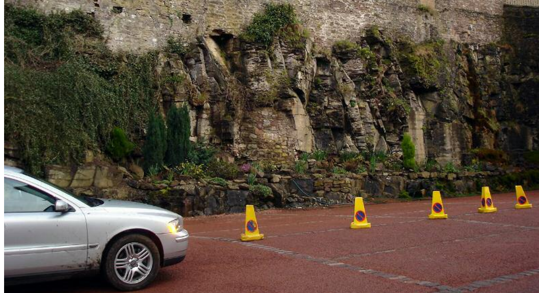
Rock slope and old masonry walls at New Lanark prior to stabilization works.
