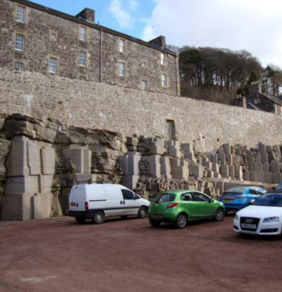
Rock slope and old masonry walls at New Lanark after stabilization works.
